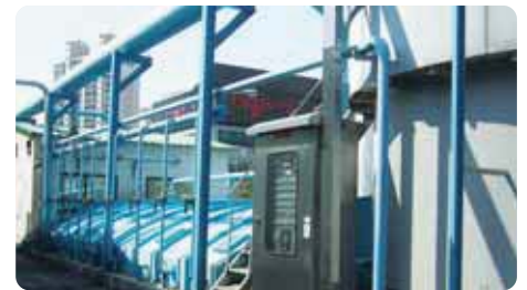
| Waste water processing facility |
