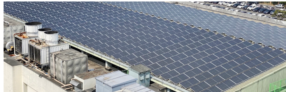
Installation of solar panel facilities at the Daepoong Factory (construction completed in November 2022)
