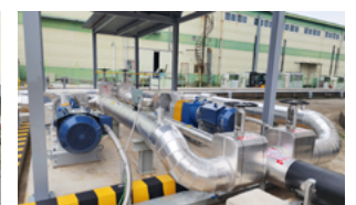
Transport oil through transfer pipes
